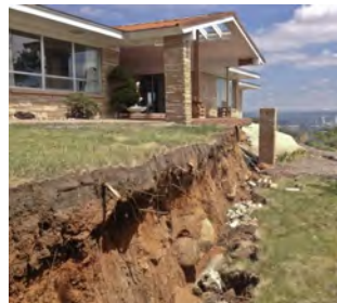
Photo: Constellation drive landslide, Colorado springs, August 2015. Source: T.C. Wait, Colorado Geological Society
